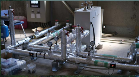
The geothermal heat pump experimental system
